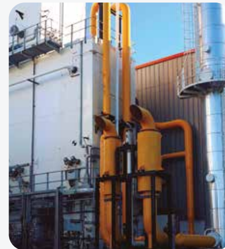
1. SMR Steam Methane Reformer
